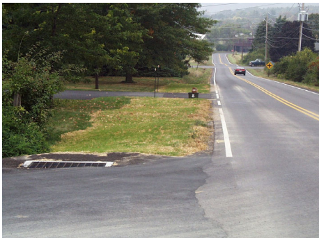
Remove the Hazard
