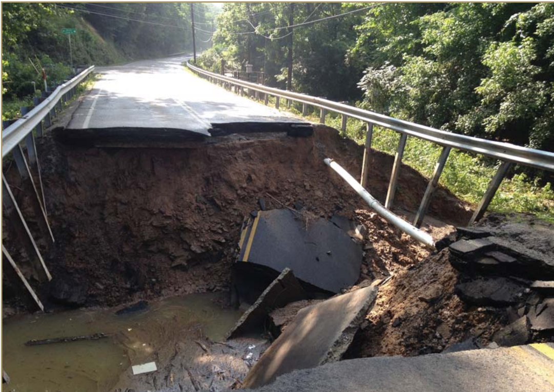
Photo by the WVDOT showing WV 4 outside of Clendenin that was damaged by the June 2016 flood.
