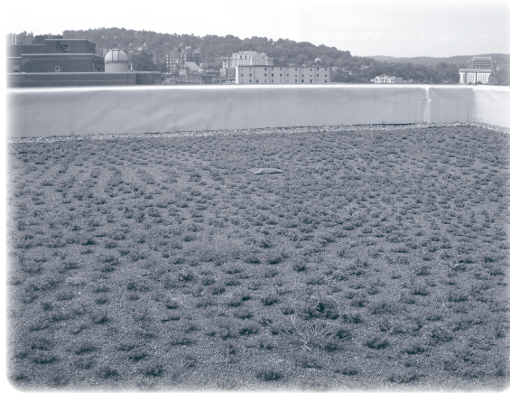
Photo of the green roof on Brooks Hall at West Virginia University.
